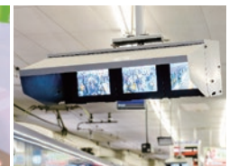
Monitoring TV system
