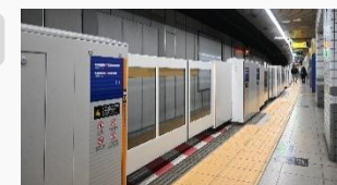
Platform screen doors
